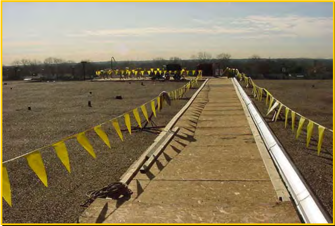
Warning Lines For Safety And Walk Way Protection
