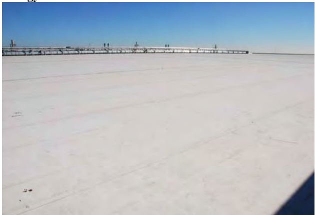
Energy Star PVC Roof
