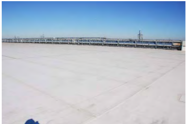
Energy Star PVC Roof
