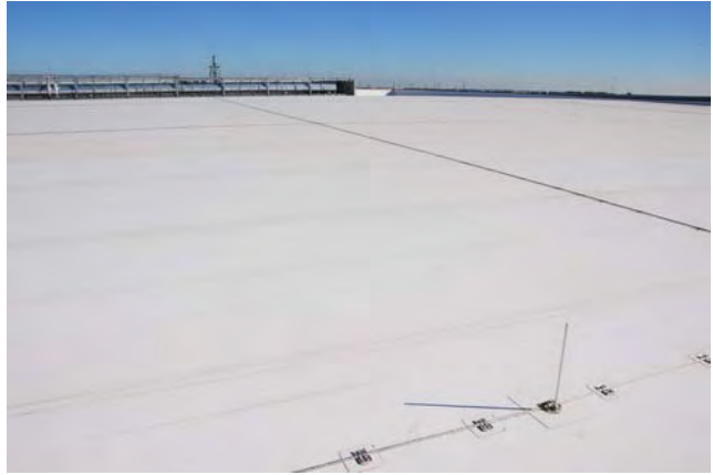
Energy Star PVC Roof
