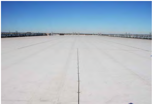
Energy Star PVC Roof
