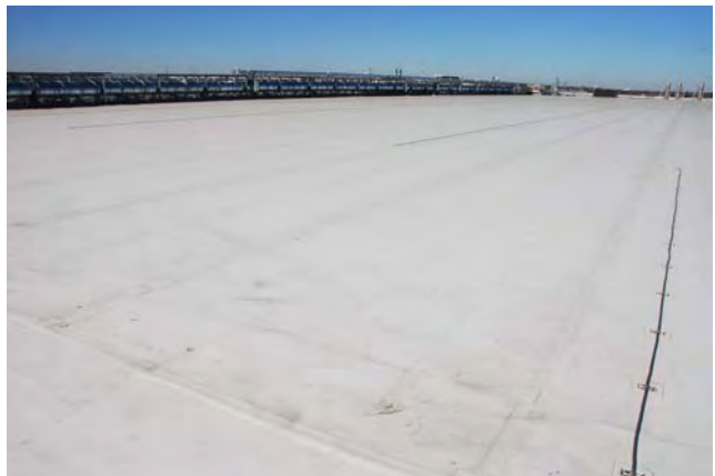
Energy Star PVC Roof
