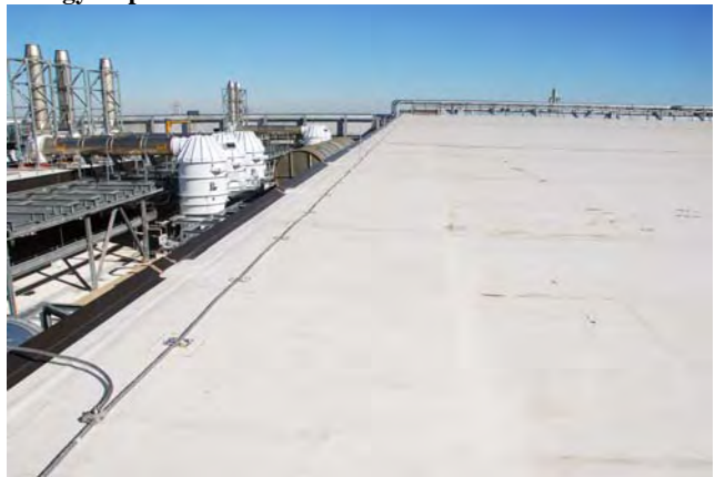
Energy Star PVC Roof
