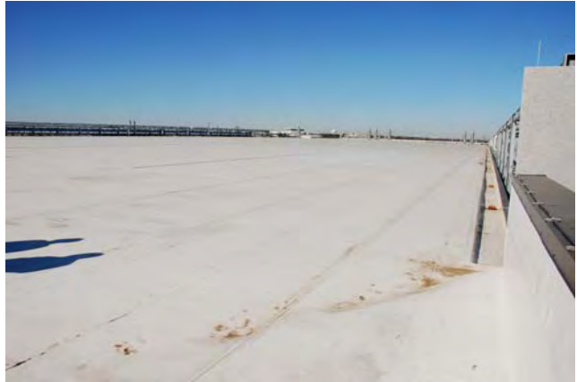
Energy Star PVC Roof
