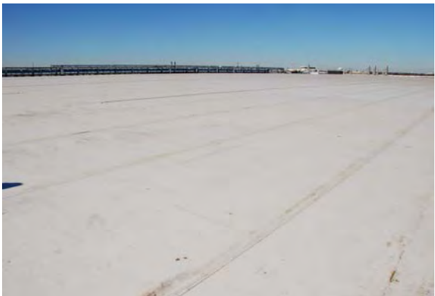
Energy Star PVC Roof
