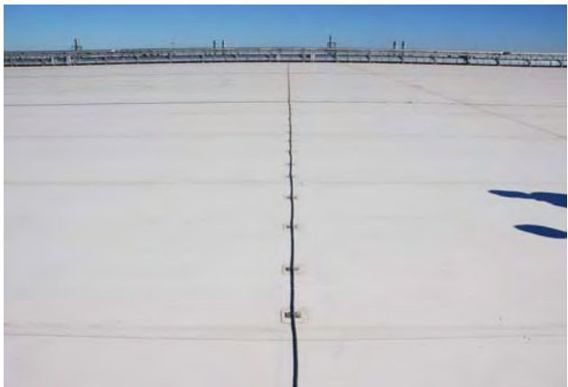
Energy Star PVC Roof
